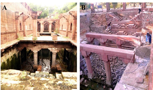
Fig. 12 a Damaged Navlakha Baori, b renovation work going on at Navlakha Baori hydro-geosite
